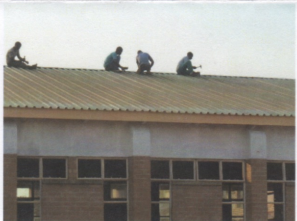
Construction team putting some finishing touches on the new classroom block, ready for Phase Two!
